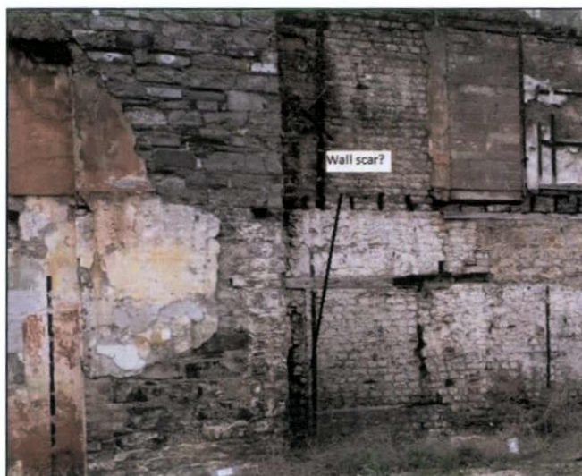
Figure 81 Wall scar of Building 2
